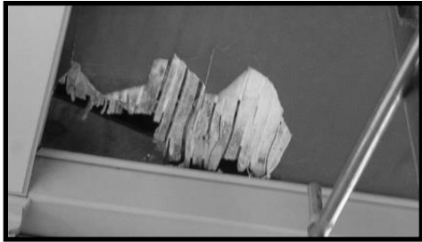
Hole in Hall ceiling.
